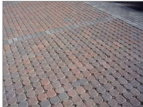
Pervious pavement that allows water to infiltrate soil.
